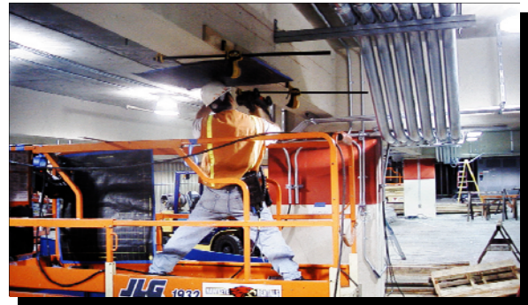
No Access to Back of Concrete
